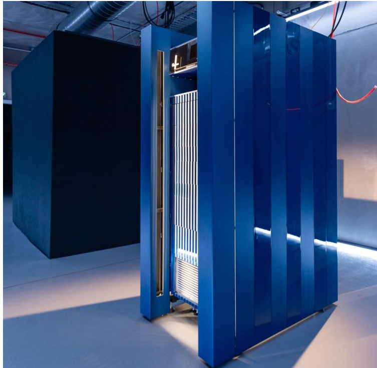
Photograph of the Quantum Processor installed at OVH-Cloud data-center in 2023 (France)
